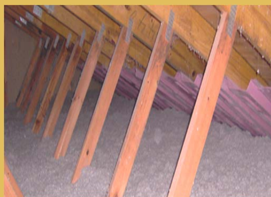
Below: An attic with blown-in T•A•P™ insulation.
